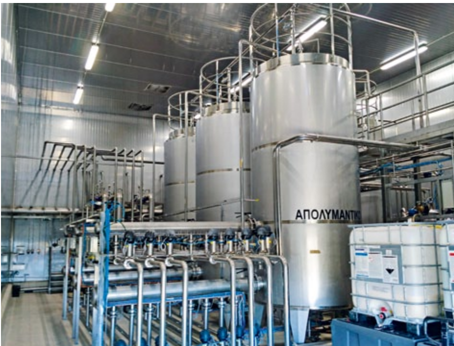
(photo: Automation System Hellas)
